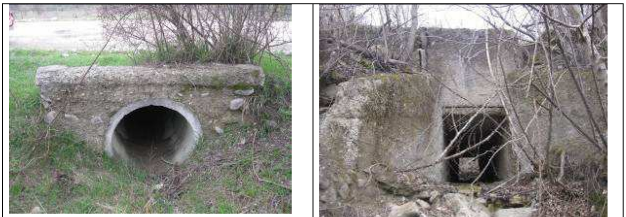
Fig.4 Current condition of culverts on the Sasadilo – Sioni Road
