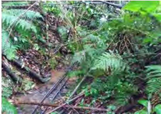
Water supply pipes from collection structure
