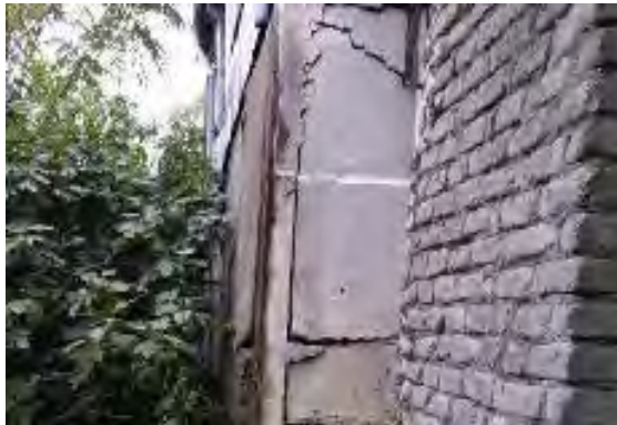
Cracked walls due to shifting soils. (41°40'45.91"N, 41°42'18.57"E).
