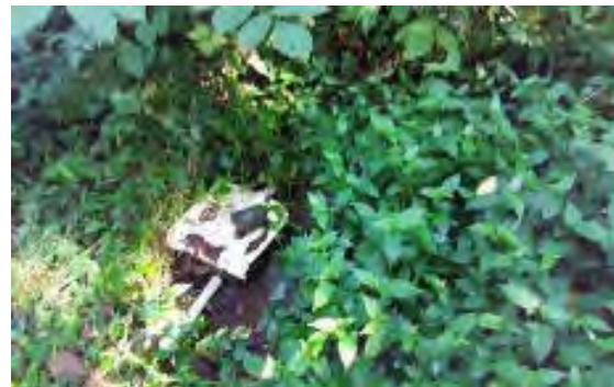
Spring water collection structure
