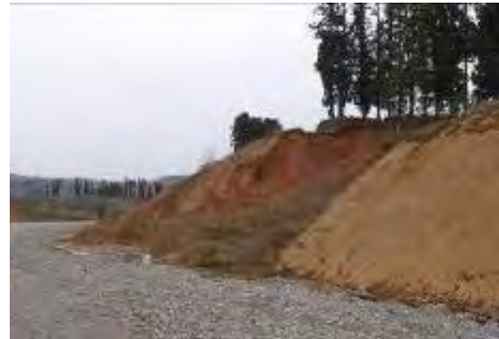
Landslide in lateritic slope at km 0+500.
