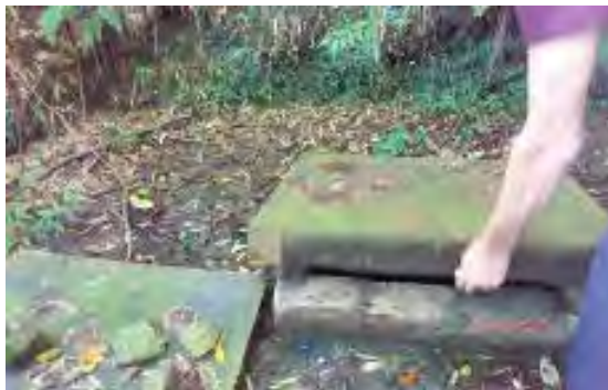
Spring water collection structure
