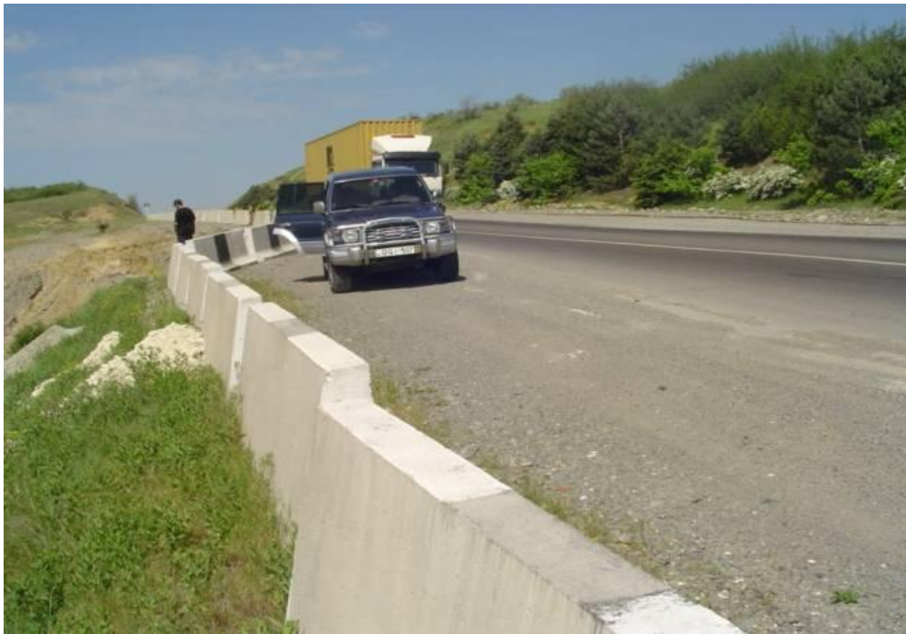
Pic. 6.1. Landslide at the Gori pass
