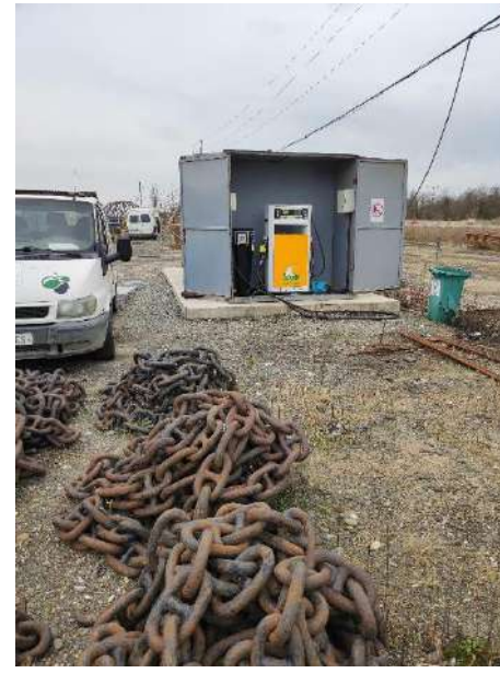
Fuel Station on Site ( with minor oil spills)
