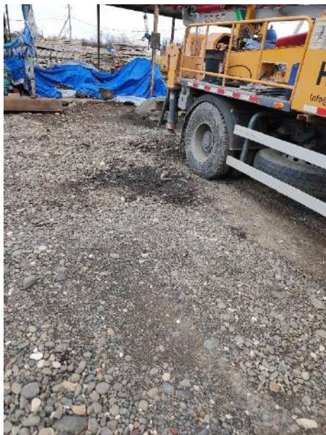
Oil Spills near unused truck
