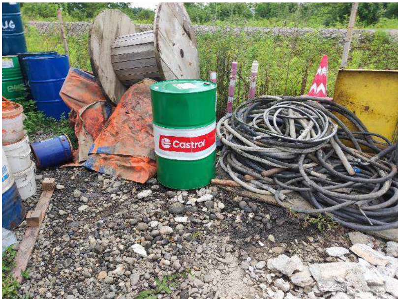
Improperly stored hazardous material
