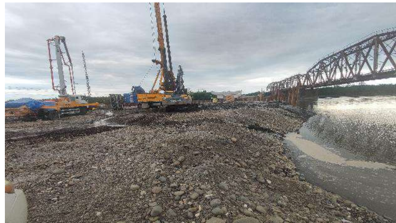
Wastewater Spill into the River from the Peninsula
