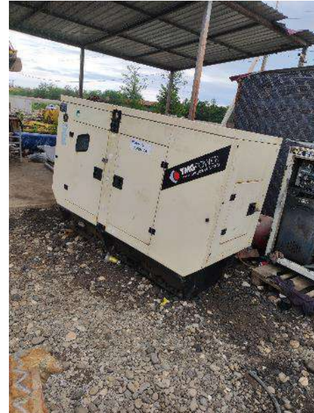
Oil spills near unused generator
