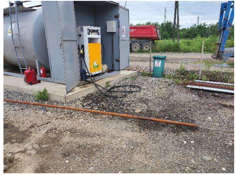
Fuel Station on Site ( with minor oil spills)
