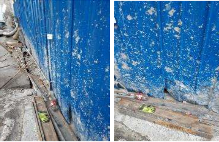
Picture 15: Non-compliance (Electrical safety) – (Workshop in Tunnel N2) – Non-compliances to H&S standards have been observed during site walk last week. It was observed that the life electric cable was passing through construction materials (Used rebar) and was pressed between steel parts. There was a big possibility that the cable could become damaged and somebody from working personnel could get electric shock there. Engineer asked Contractor’s site responsible person to switch off the power, remove the cable, elevate it and fix it on a safe height to avoid possible incidents. After some time, cable was disconnected from the power supply, collected and redirected by using safer route. Issue closed.
