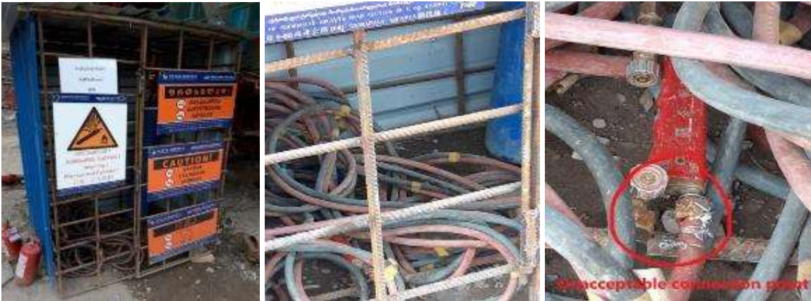
Picture 9: Material storage (Possible incident) Tunnel N2 – Engineers are still observing issue related to improper storage of materials at workplaces. Such case has been observed during visiting the tunnel N2. The rubber hoses, using for connecting the propane cylinder to heating torch has been found stored in the same cage with the oxygen cylinders. Also, handmade connections have been found during site inspections. Site responsible person from the Contractor Company was informed about it by the Engineer. The Engineer asked to keep all mentioned above materials separately, especially arranged for such materials designated places. Issue open.
