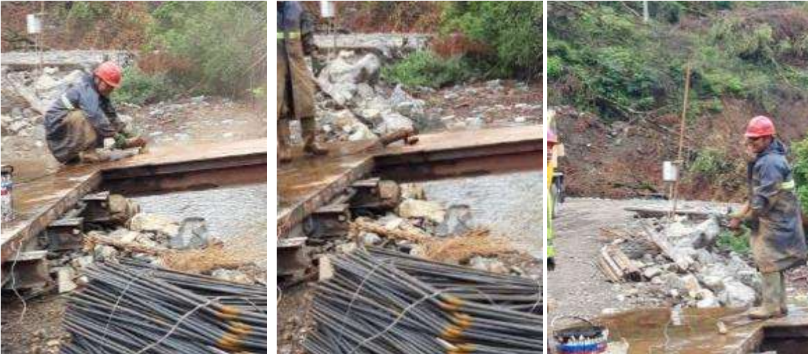
Picture 27: Non-compliance (Personal protective equipment) – Bridge N2, pier#5 – Non-compliance to health & safety rules and requirements have been observed during visiting the workplace. One of the Contractor’s personnel was using brushing machine to clean the steel plate surface and he didn’t use the safety glasses to protect his eyes from possible injury. The Engineer asked him to stop, wear safety glasses and then continue performing the task. The worker wear his safety glasses on and continue performing the task. The responsible persons from the Contractor Company were informed about it. The Engineer asked them to do workplace inspections very often to find out and eliminate all possible risks of getting injury. Issue closed.
