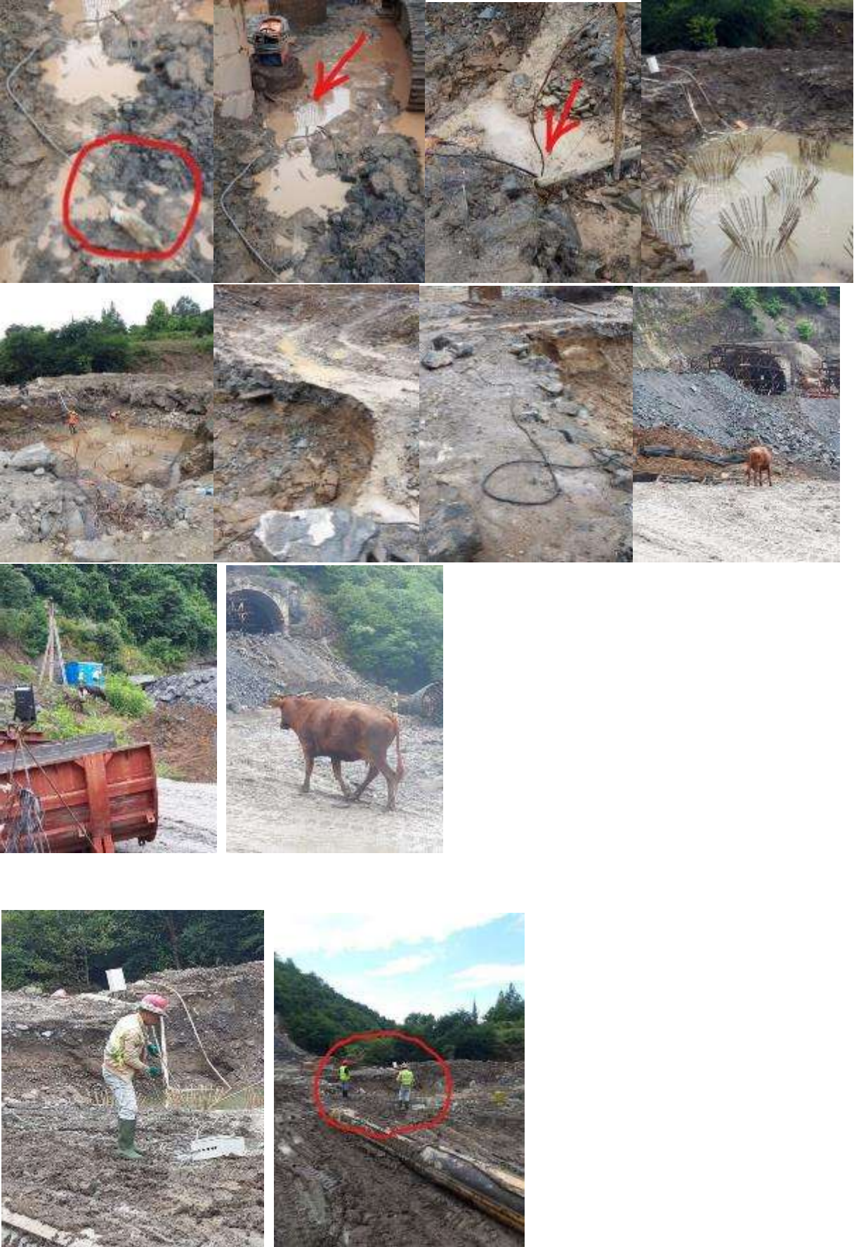
Electric cables removed from the water and fixed in the isolated box.
