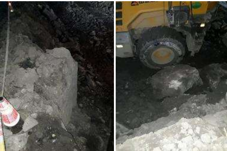
Picture 28: Non-conformance– (Possible personal injury) - (Tunnel #3 TA) – The cracked piece of big rock has been observed inside the tunnel (Pandus - access road for the drivers). Any time, because of possible vibration, it could become loose, roll down and injured somebody. The Engineer asked the loader operator to demolish this rock and remove it out from the tunnel to avoid possible injuries of working personnel. The Engineer asked responsible persons from the Contractor Company to be more attentive and do everything is necessary there to avoid such situations at workplace. Issue closed.
