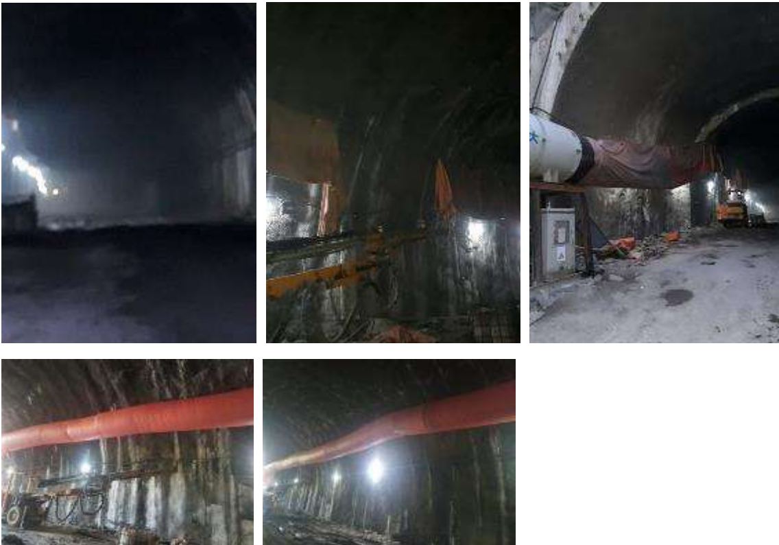
Picture 22: Non-compliance (Poor ventilation-Possible injuries) -Tunnel #2AT- Non-compliance to H&S regulation has been observed during site inspection of tunnel #2. The level of oxygen was very low due to a destroyed ventilation fan (the level of oxygen was tested by tester). Engineer decided to stop the work, because the working personnel, involved in the task inside the tunnel, could get hurt and be injured there. Responsible persons from the Contractor Company were called to site and Engineer has explained that due
