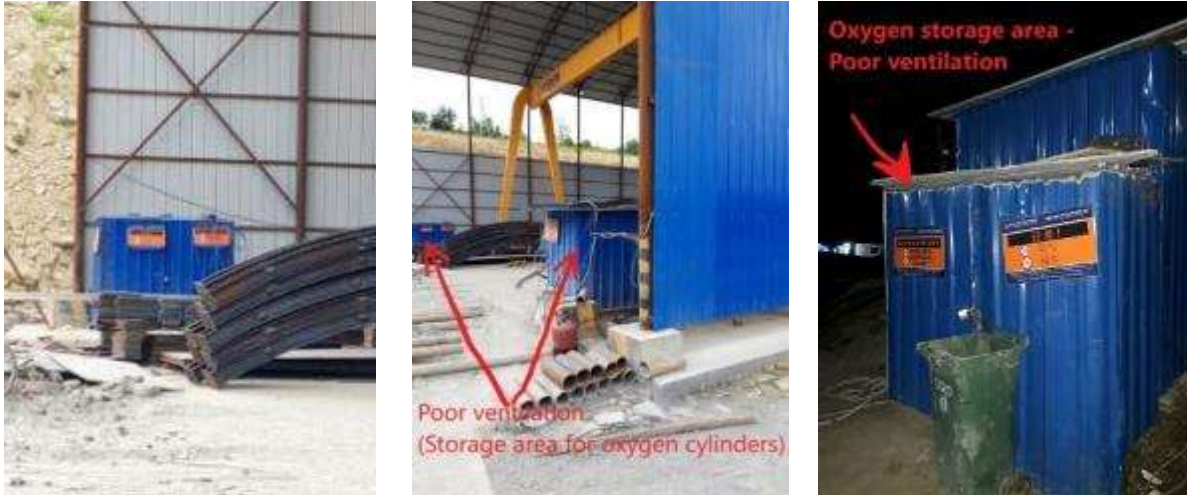
Picture 5: Non-compliance (Tools and equipment (Possible damage)) – (Tunnel N5) – Non-compliances to H&S regulations and requirements have been observed during site visit: Storage cages (To store the oxygen cylinders) aren’t equipped with proper ventilation system (Cages are fully closed). It may cause possible incidents. Engineer asked Contractor’s site responsible persons to react on mentioned above issue as soon as possible, to avoid possible injuries or property damage. Issue still open.
