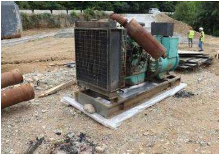
A drip Tray provided for the Generator
