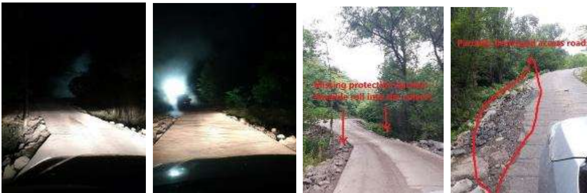
Picture 6: Driving safety (Road related incidents) – Access road to Tunnel N5 TA – It is unsafe to drive on access road to tunnel N5, because of poor road quality. It is double danger, when driving in the night time (In some section the road is becoming very narrow and there is a big risk to lose the concentration, drive out the road and turn over. In some section, road is partially damaged). Engineer asked Contractor’s site responsible persons to arrange some jersey barriers or flashing safety poles, place it on most dangerous areas of mentioned access road and protect unsafe sections and safe people’s life. Waiting for feedback, but there aren’t any updates until now. Issue open.
