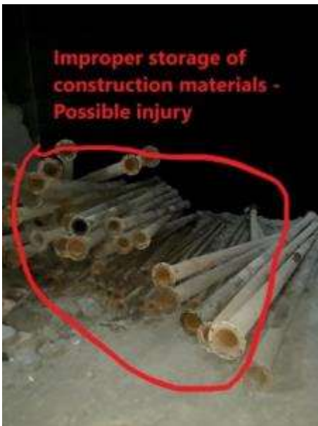
Picture 16: Improper storage of materials (Personal injury) Tunnel N3 – Violation to Company H&S rules has been observed by the Engineer during visiting the tunnel N3. It was observed that construction materials weren’t stored properly. Somebody from working crew may become stuck between the rolled pipes and become injured there. Engineer asked Contractor’s site responsible person to pay more attention on workplace safety to avoid possible incidents from happening. Engineer is waiting for feedback from the management of Contractor’s team. Issue open.
