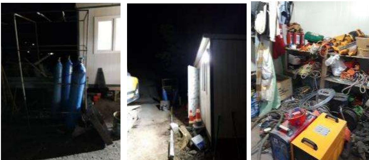
Picture 8: Non-compliance (Workplace safety) – Tunnel portal N 4004 TA - Mostly all health & safety related issues were solved on mentioned location, but there are some problems should be paid additional attention on. For example: Arrangement of bio toilet at workplace and improper storage of oxygen cylinders
