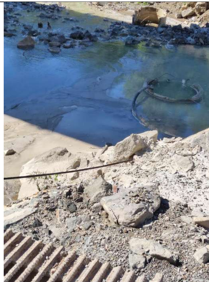
Poor Riverbed Protection and Improper water Usage (Bridge 3, August 2024)
