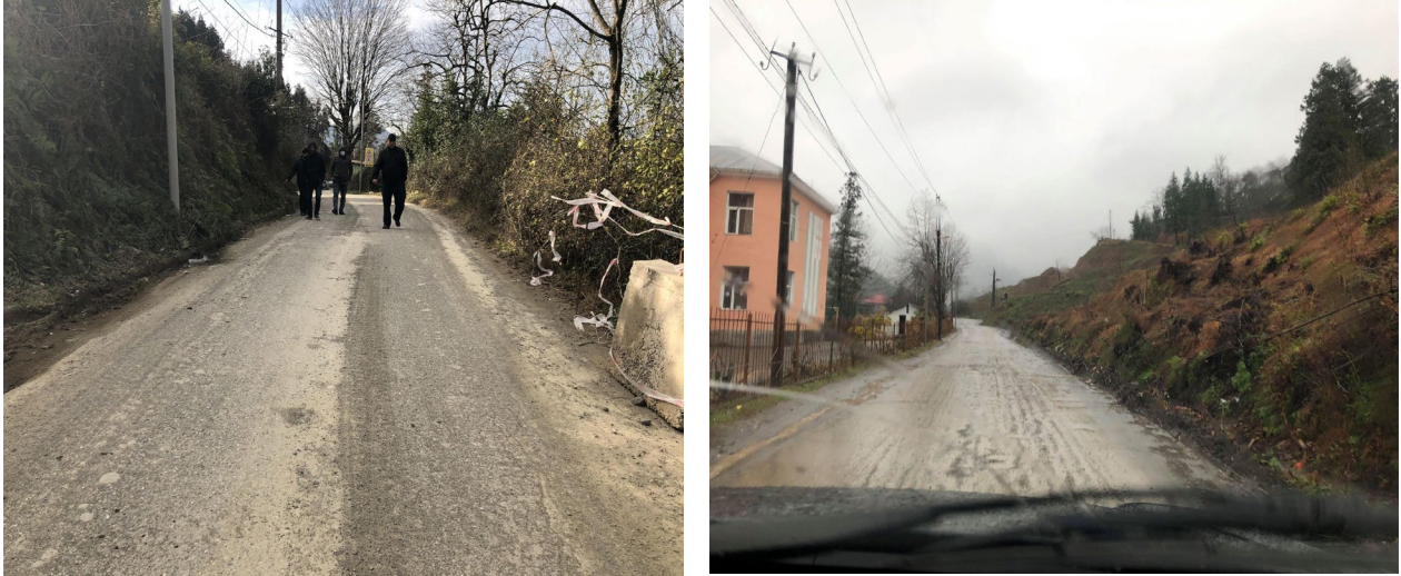
Condition of access road in dry weather and rainy day
