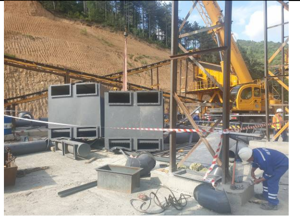
Collapsed dust collector
